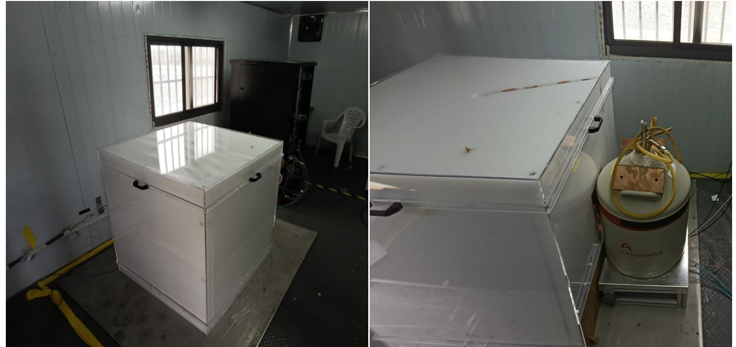
Muon detector units waiting for installation @in the container outside the containment of Sanmen NPP
